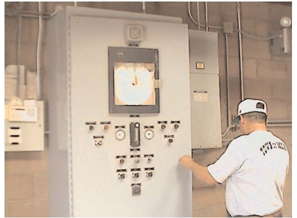
CDBG funds were utilized in the City of Miami's upgrade of its electrical plant.
