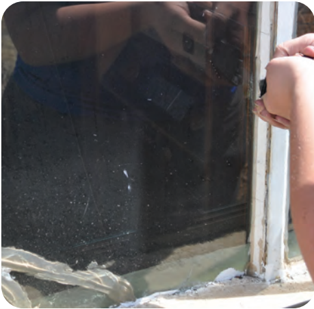
1. Remove all broken glass
