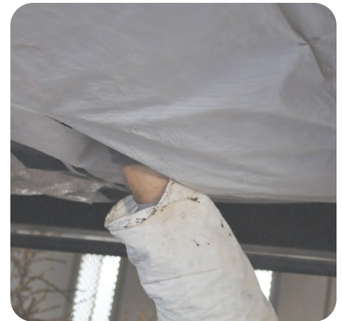
4. Cut access holes to ensure entire cavity will receive continuous and consistent insulation
