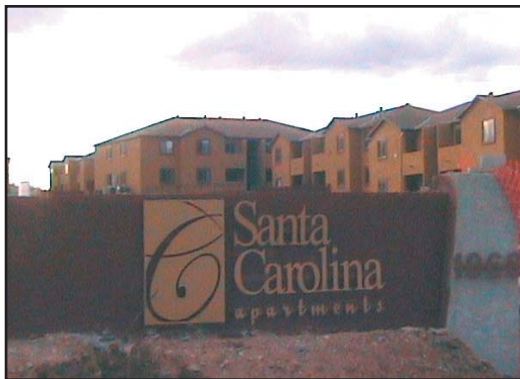
Work on Santa Carolina Apartments in Nogales nears completion. The project was financed using multi-family bonds issued by the Arizona Housing Finance Authority. A grand opening is scheduled for early May.
